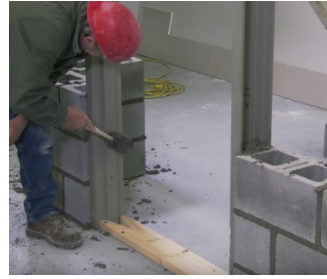
Figure 11 – Mason checks plumb level and square before laying block and throughout process
